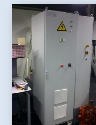
TRIPHASE Re-programmed inverter
